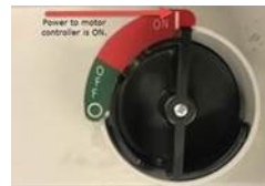
Figure 27 - Local Disconnect in On Position
